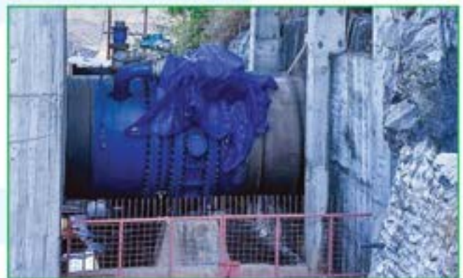
Penstock Protection Valve House
