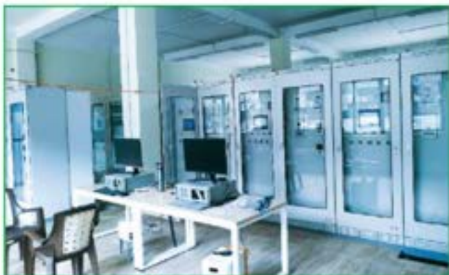
Control Room in powerhouse
